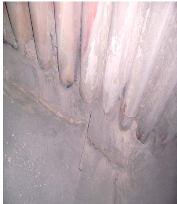
Photo 4: Ash waterwall roof panel inside penthouse. Wherever the cracks are there, the air gets inside.
