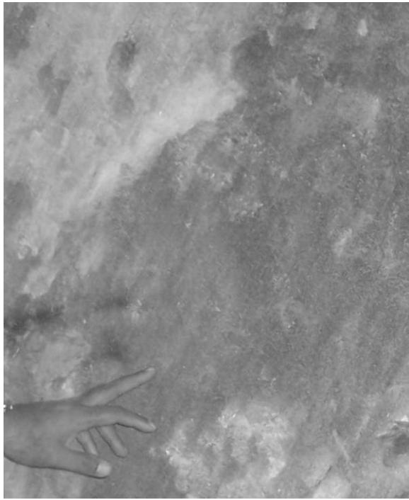
Photo 1: Furnace ash deposits in bio mass due to high furnace temperature
