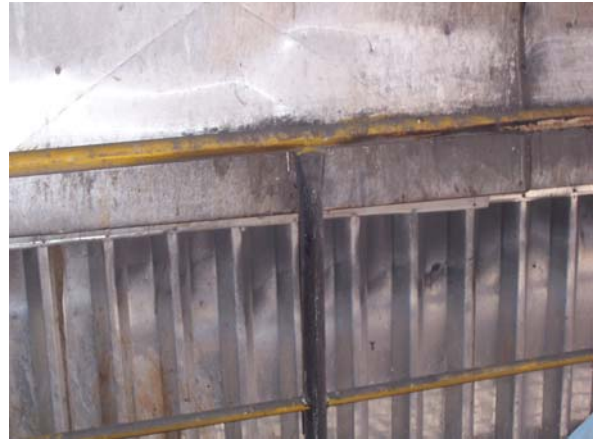
Photo 6: Indications of smoke at penthouse confirm air ingress. When the furnace pressure goes positive at times, the flue gas comes out.
