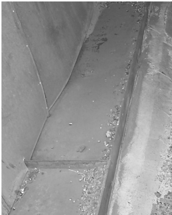
Photo 3: Fresh ash spills around leakage points in roof seal box
