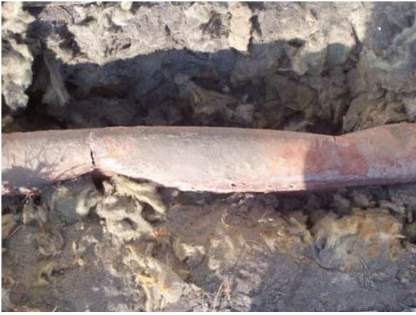
Photo 5: The failed metallic expansion joint is seen after removal of insulation cladding at Economiser inlet duct. Such leakage locations lead to wrong to O 2 indications.
