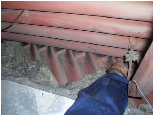
Photo 7: Indications of dust below waterwall nose panel. The seal was not done as per drawing.
